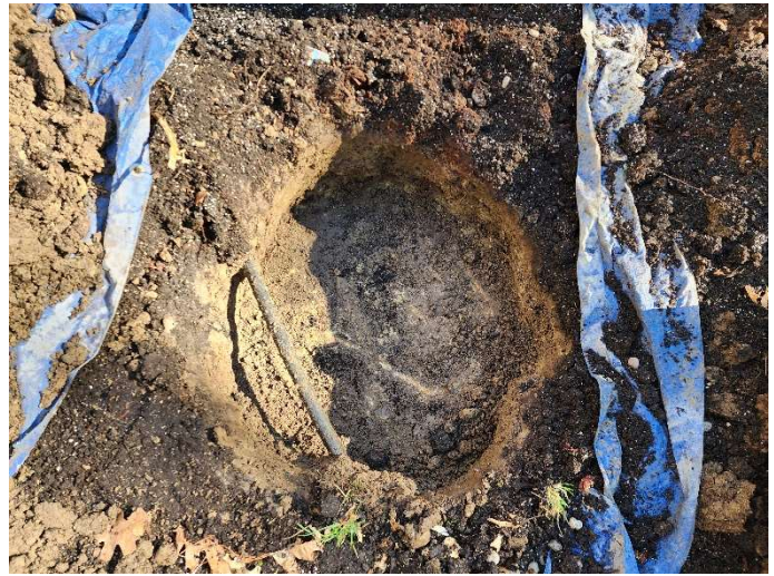
Picture of outlet cover before opening
