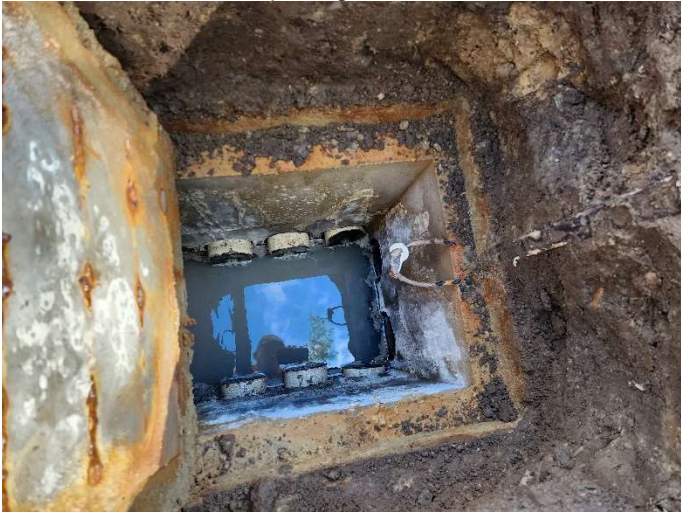
Picture of distribution box after opening
