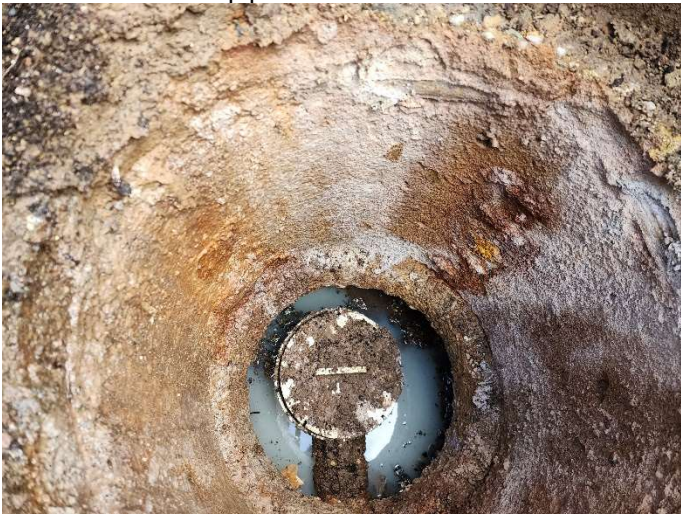
Picture of filter in place but not cleaned
